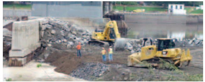
This picture, taken September 23rd, shows massive effort to close the breach around the dam at Lock 8/Maalwyck Park
