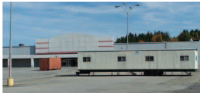
Former Kmart store to make way for Target - Asbestos removal underway, with demolition to follow in November.
